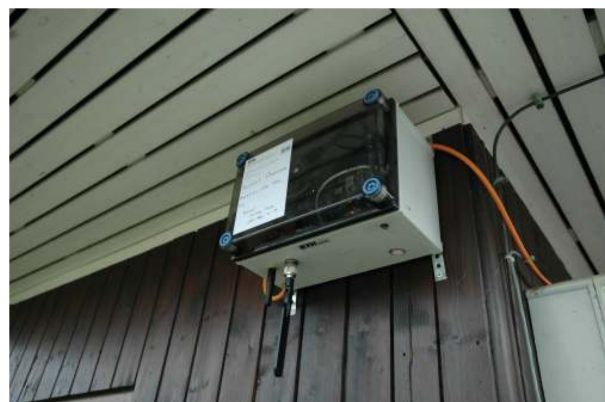
OpenSense node placed next to the NABEL station Duebendorf for initial calibration
